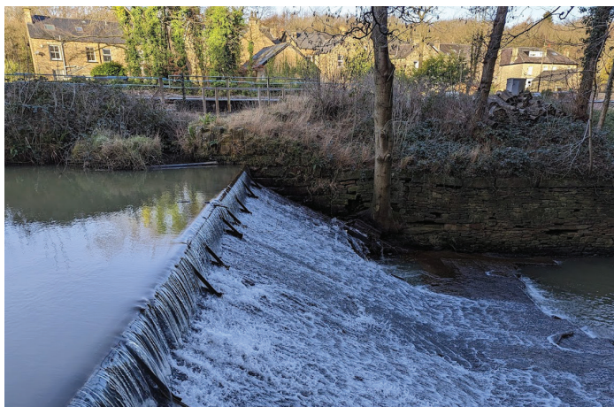
The weir on the Sheaf with sluice on opposite bank. Houses are on Abbeydale Road South, railway in between. (Photo: Roger Hart)
